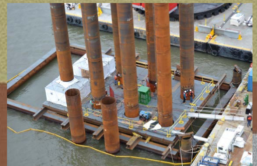
Once driven deep into the soil beneath the riverbed, these steel-pipe piles will be filled with steel-reinforced concrete.
